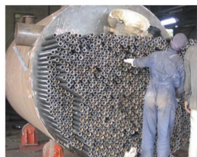
Tubes in a heat exchanger
